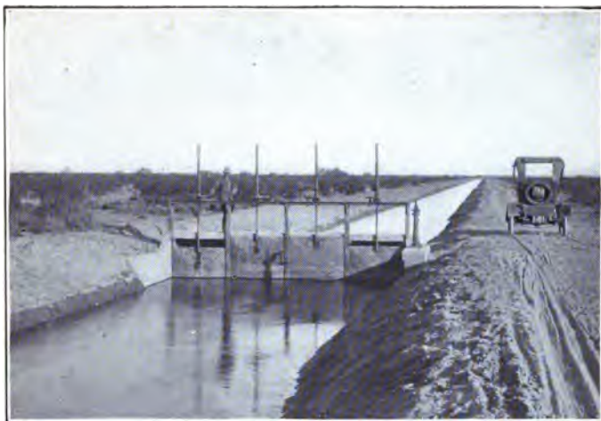
CONCRETE AND STEEL GATES IN EARTH CANAL, PERMITTING REGULATION OF WATER.
